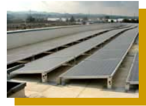
PV Panels at IEUA Headquarters
