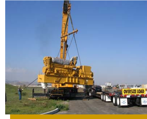
1.5MW Caterpillar Engine at RP-5
