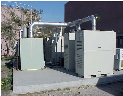
Picture below: Microturbines
