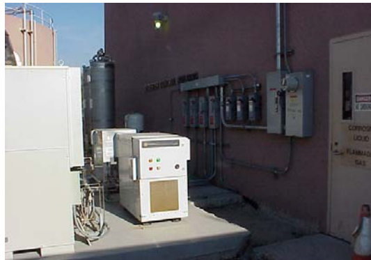
Picture above: Microturbine disconnection switches
