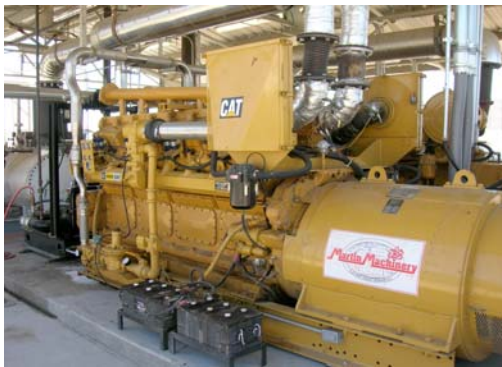
Picture above: 400 kW reciprocating engine
