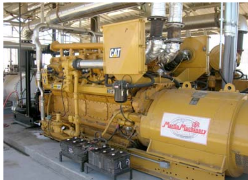
Picture above: 400 kW reciprocating engine
