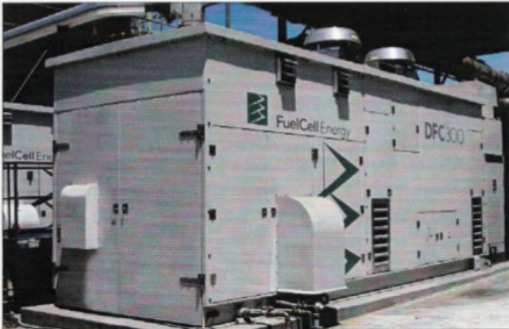
500 kilowatts of Ultra-Clean Direct FuelCell® Power
